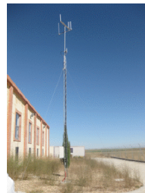
Remote controller outside the pumping station
