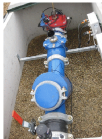
Hydrant in the field
