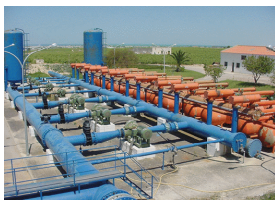
Pumps, filters and hydroneumatic tanks
