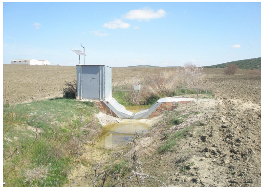
Figure 4 Hydrological station for monitoring irrigation return flows at the Genil-cabra irrigation scheme, Spain
