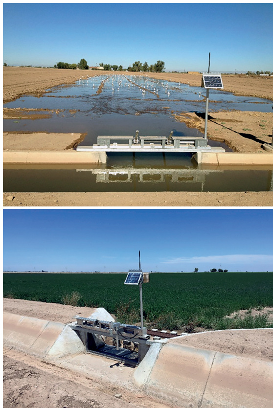
Figure 2. Surface irrigation automated gates in Holtville, California.
